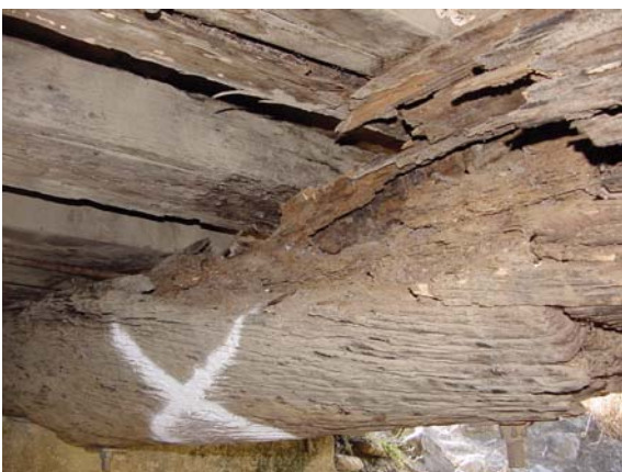
Figure 2 Bridges in need of risk management strategies.
