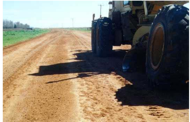
Photo 3.12 – Conventional Flat Blade. Note the smoothing of the surface which tends to occur and the poor mixing and spreading of the material. Also note the width being worked and relatively flat formation
