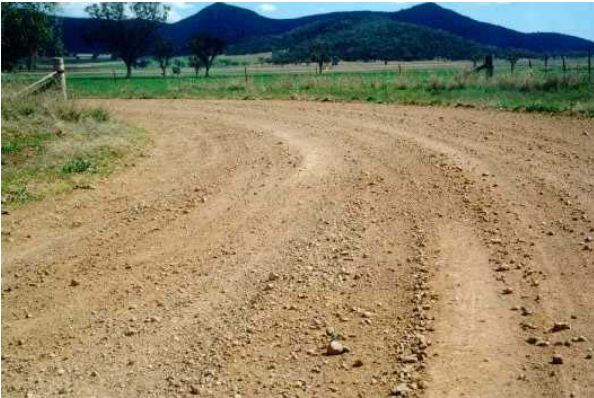
Photo1 – Bulga Road. Note the amount of loose material on the bend and the large rocks left after the fine material is lost either to the sides or as dust
