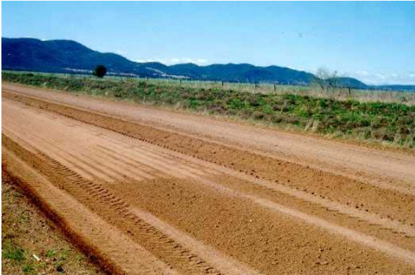
Photo 3.10 – Breeza – Piallawa Road. Shows the point at which the free-roll is applied to the graded road. Note the greatly improved surface due to this compactive effort
