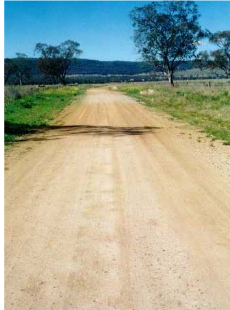
Photo 3.9 –Coochooona Road. Shows the use of patching to keep the road serviceable. Note the potholes due to a flat formation and lack of compaction at the time of placement
