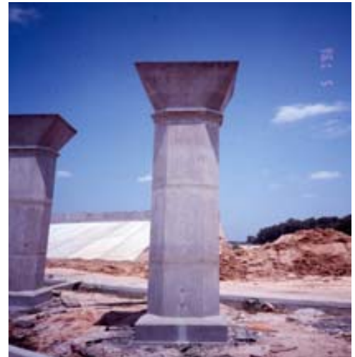
Segmental Precast Concrete Pier
